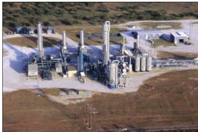
Enterprise Products owns and operates the Thompsonville gas plant south of Hebronville, Tex. The recently expanded to 330-MMscfd turboexpander NGL recovery plant was built in 1993 by Optimized Process Designs Inc., Katy, Tex. It employs advanced control strategies for gas processing rate management as well as automatic composition control of the demethanized product. Photo from Enterprise Products.
