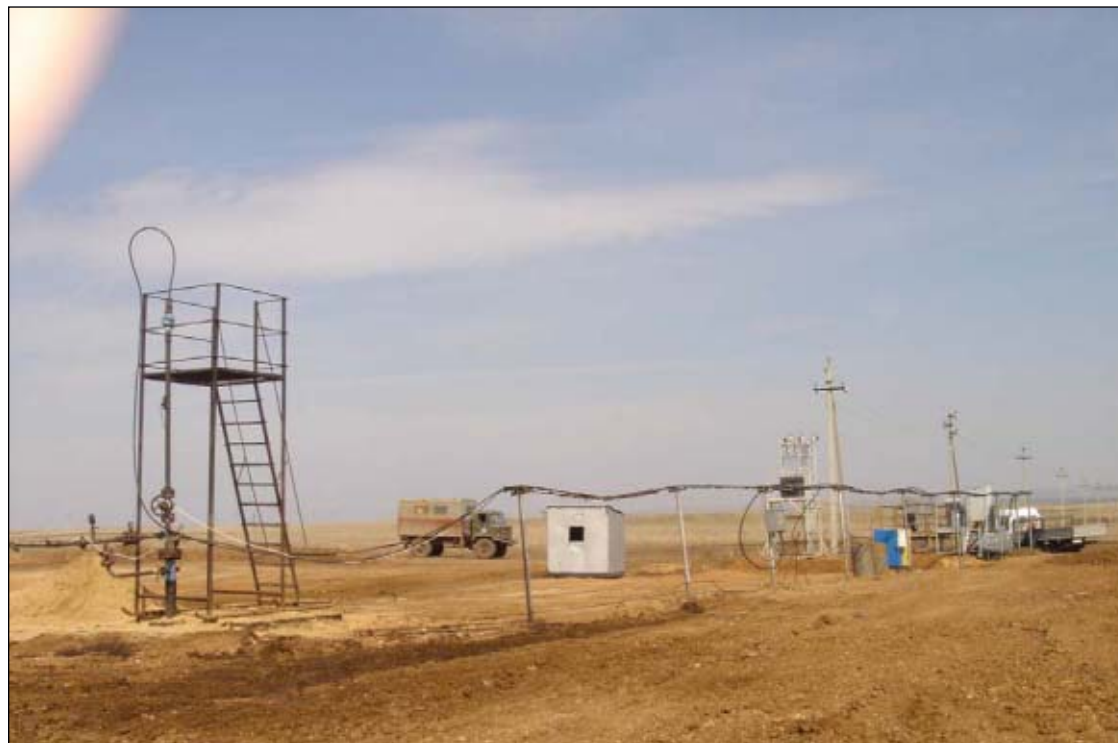
The heating system includes the cable in the well and associated control equipment (Fig. 1; photo from Nefteservis-NN).
